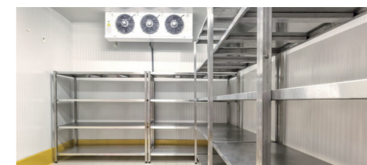
Restaurant cold rooms
